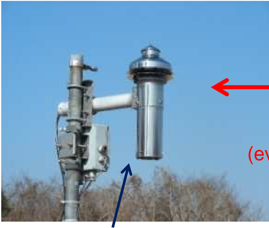
Ventilated shield Electric thermometer Electric hygrometer
