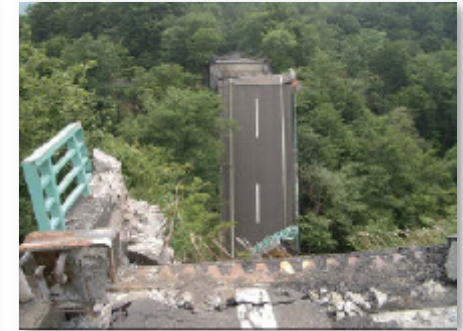
▲The Iwate-Miyagi Nairiku Earthquake in 2008
